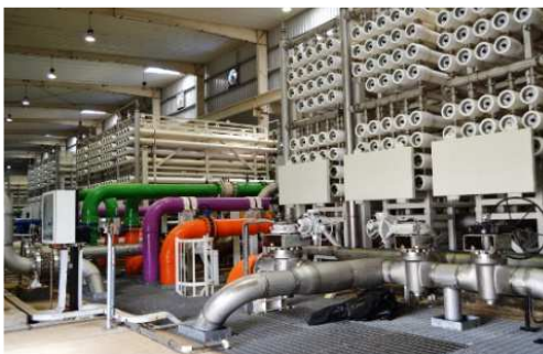
□ Ultrafiltration and reverse osmosis desalination plant in Accra (Ghana).
