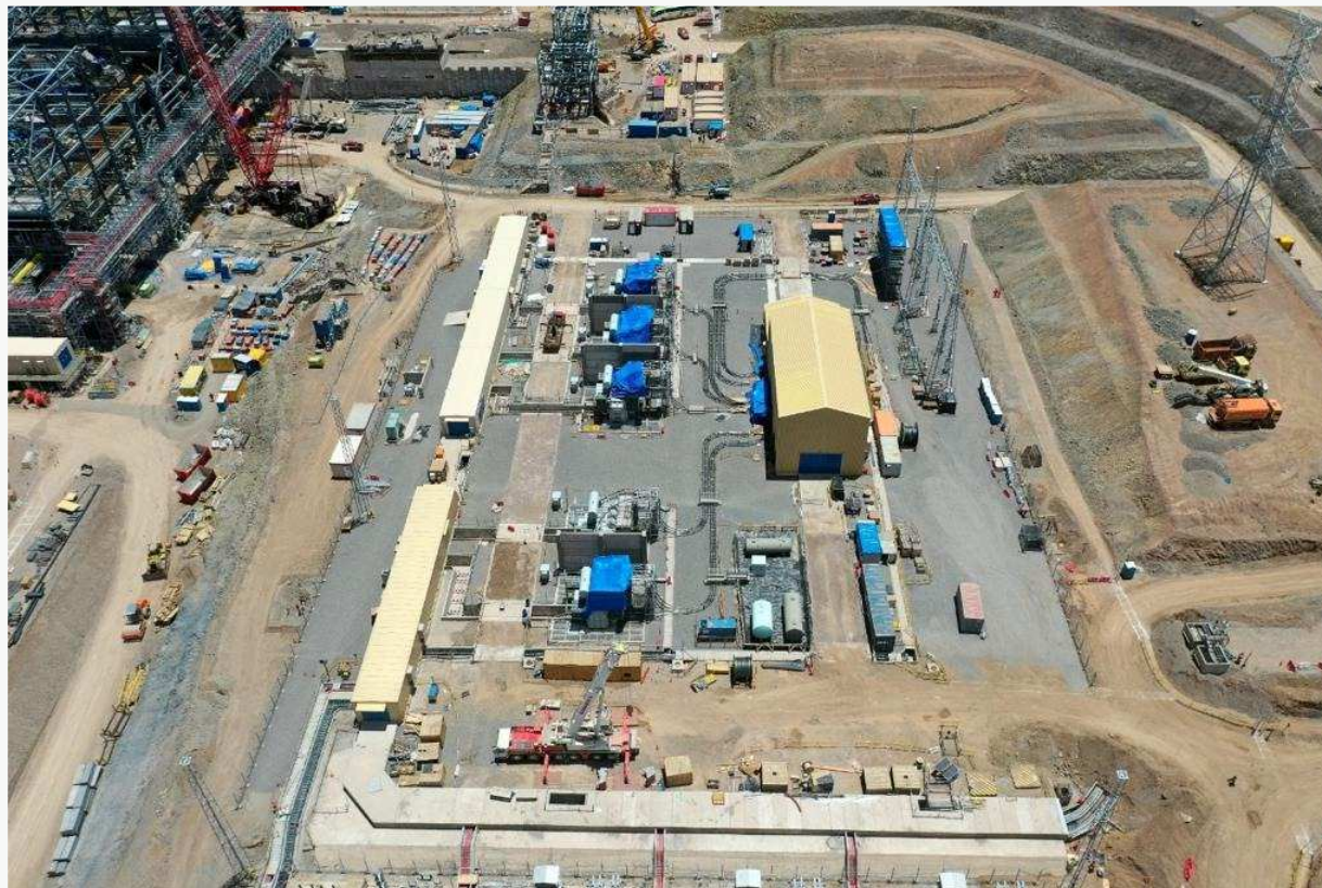
□ Electric substation for the second phase of the Quebrada Blanca mine in Chile.
