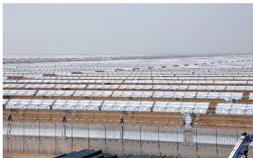
□ Support structures for parabolic trough collectors at the Mohammed Bin Rashid Al Maktoum plant.
