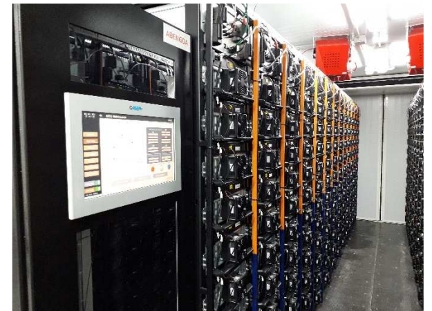
□ Inside the BESS container, showing the battery racks and the local control box at the front.
