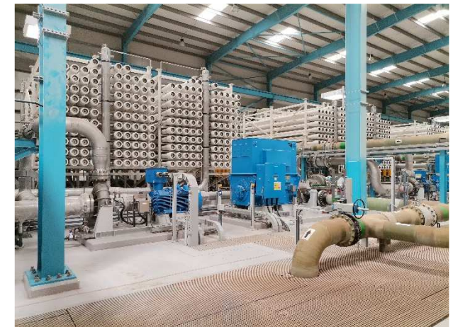
□ Desalination plant in Salalah, Oman.
