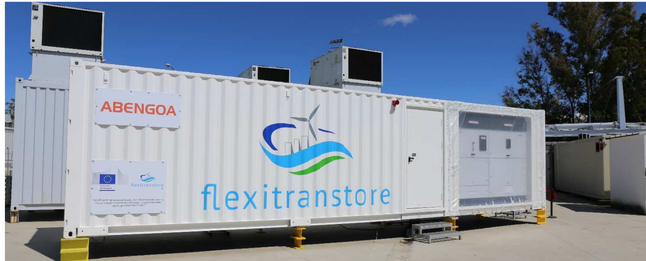
□ BESS container installed at the Athienou substation (Cyprus).
