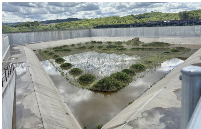
Retention pond at Nozomi
