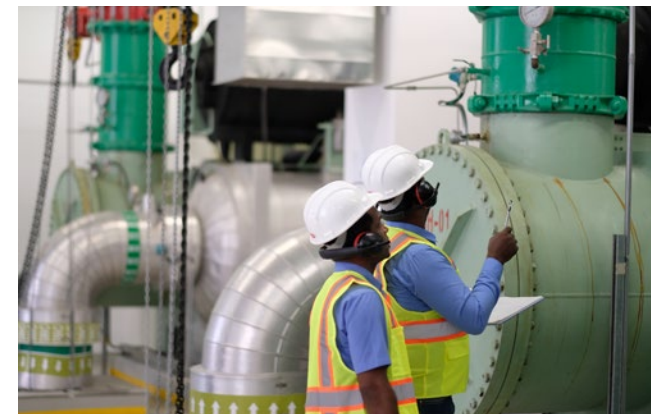
Cooling systems at Emicool
