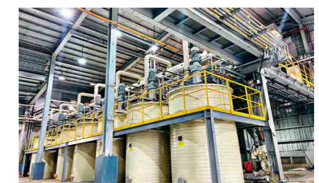
LIANYOU METALS’ solvent extraction equipment
