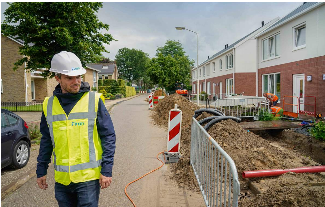
In 2024, we worked on developing and expanding district heating networks in various municipalities through our subsidiary Firan.
