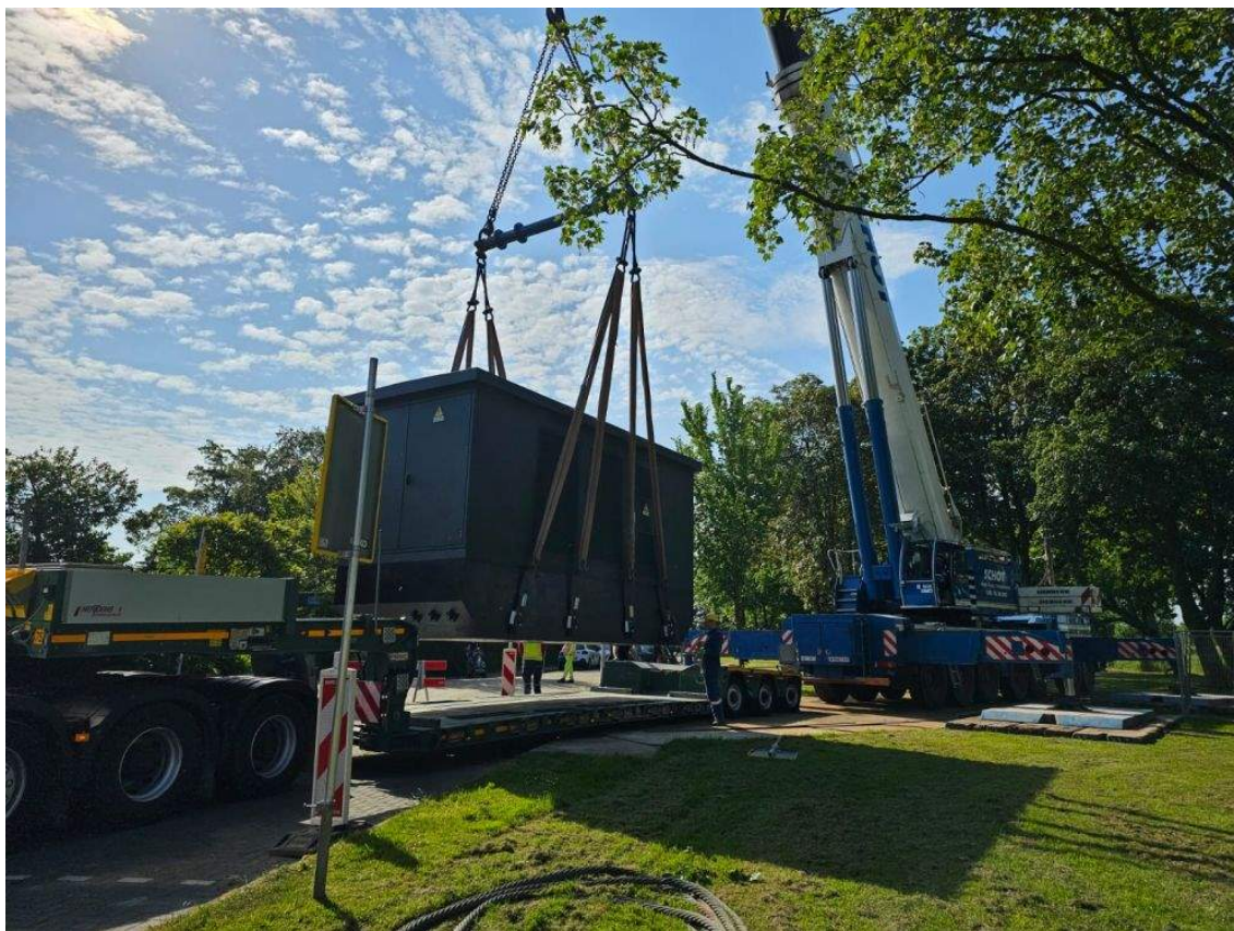
The Liander Netuitbreiding Lelie programme (abbreviated as NuLelie) is an amalgamation of many projects. We are laying over 3,000 kilometres of electricity cables and installing or modernising over 400 electricity substations.
