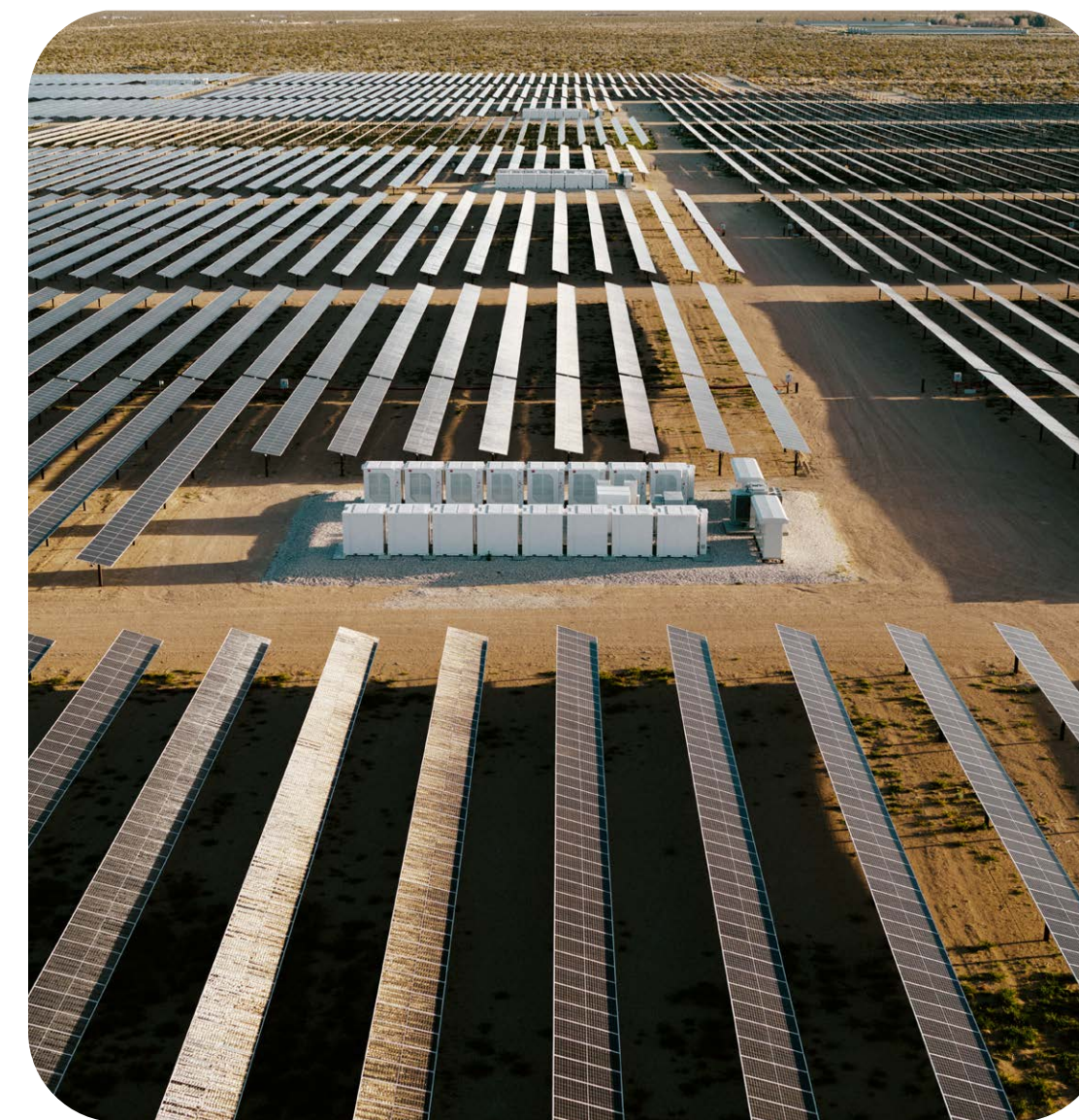
The Baldy Mesa Solar and Storage Project in Adelanto, California (developed and operated by AES), represents one of the solar projects that we added to our portfolio that includes storage capacity.
