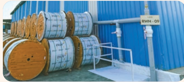
Rainwater collection from roof-top at APAR's Khatalwada plant.
