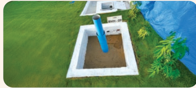
Filtration chamber filled with filtering media such as fibre, coarse sand and gravel layers to remove debris and dirt from water before it enters the recharge structure.
