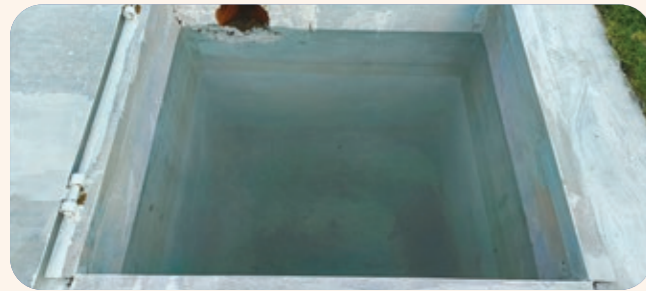
Silt trap (sediment trap or sediment basin) Chamber -- used to capture and filter out sediment and other pollutants from rainwater before it enters the ground to ensure water quality and comply with environmental regulations.
