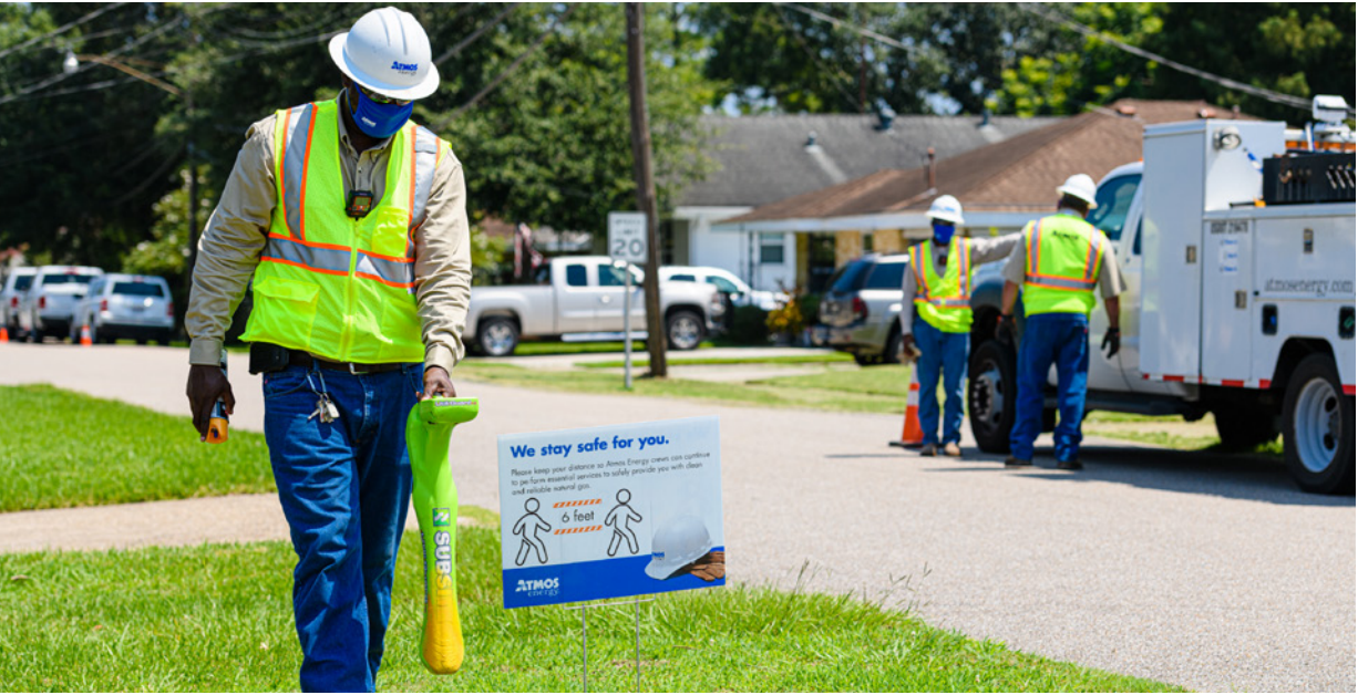
Calling 811 to locate and mark utility lines is crucial for safe digging. Clem, a Crew Leader, marks a natural gas line with temporary paint in Louisiana.
