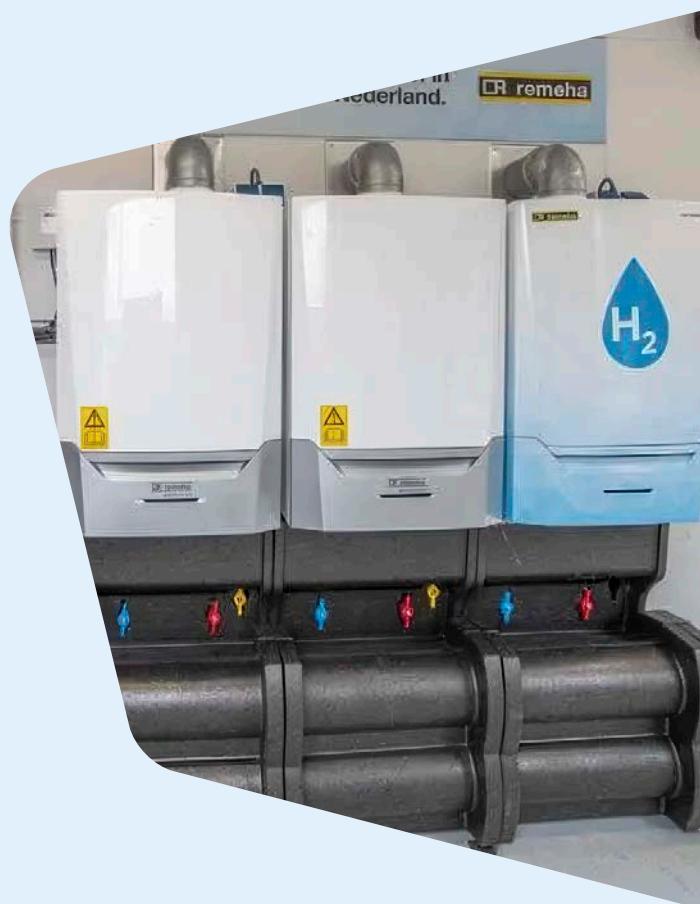
Commercial hybrid system with 100% hydrogen boiler
