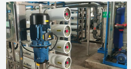
Yanjing Brewery Reverse Osmosis Water Secondary Treatment Project
