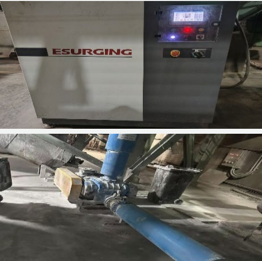
Solid Waste Treatment Platform's Innovative Sludge Co-incineration Technology
