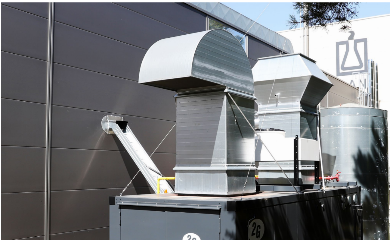
CHP station at BRAND KG
