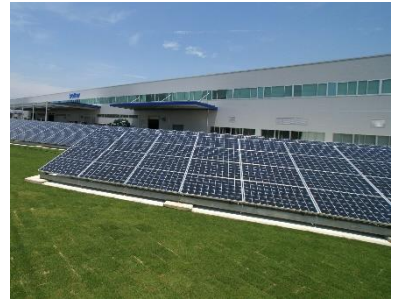
Solar panel in Kariya Factory
