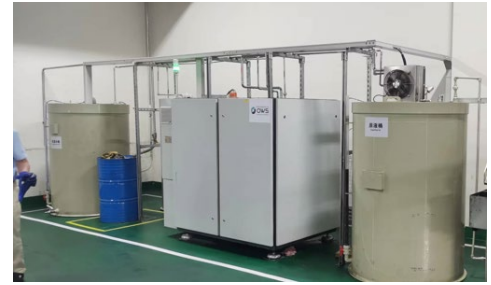
Brother Machinery Xian Co., Ltd.: Waste liquid treatment system
