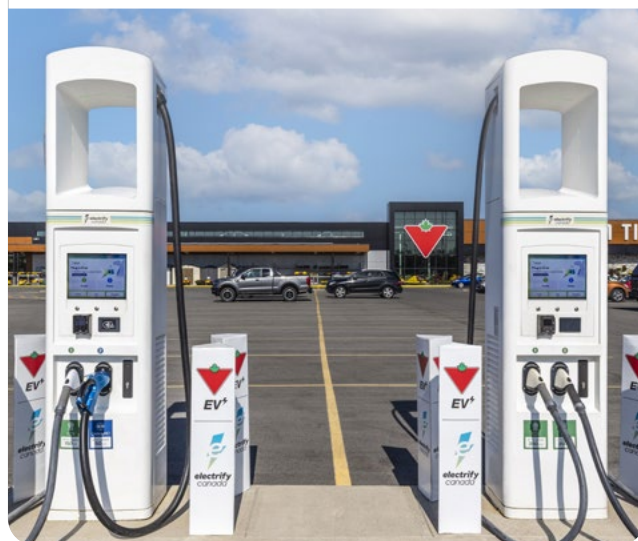
Electric vehicle charging stations at a Canadian Tire Store – Welland, Ontario
