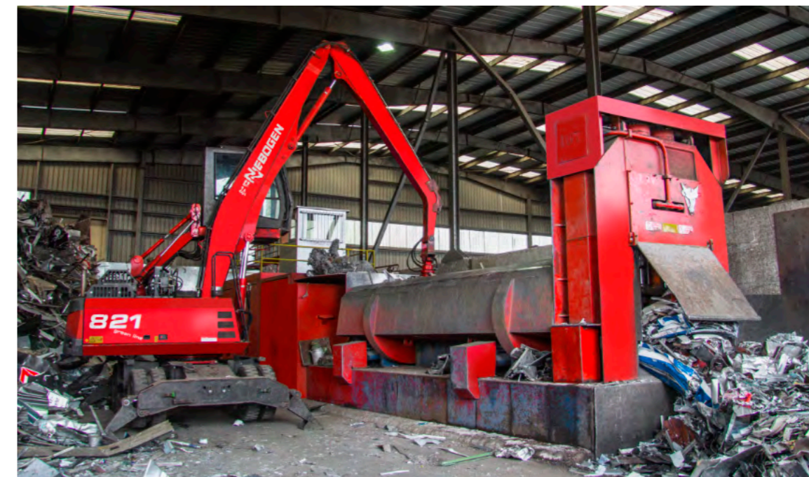
The scrap shear treats the scrap through chopping to a chargeable size.
