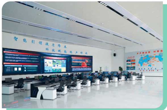
Intelligent Central Control Room
