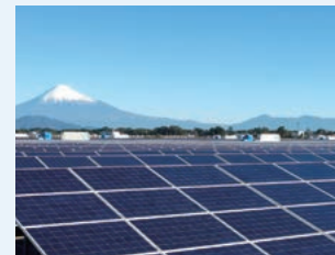
Mega Solar Shimizu (2015)
