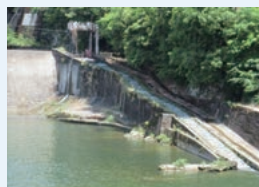
Fishway installed in a dam
