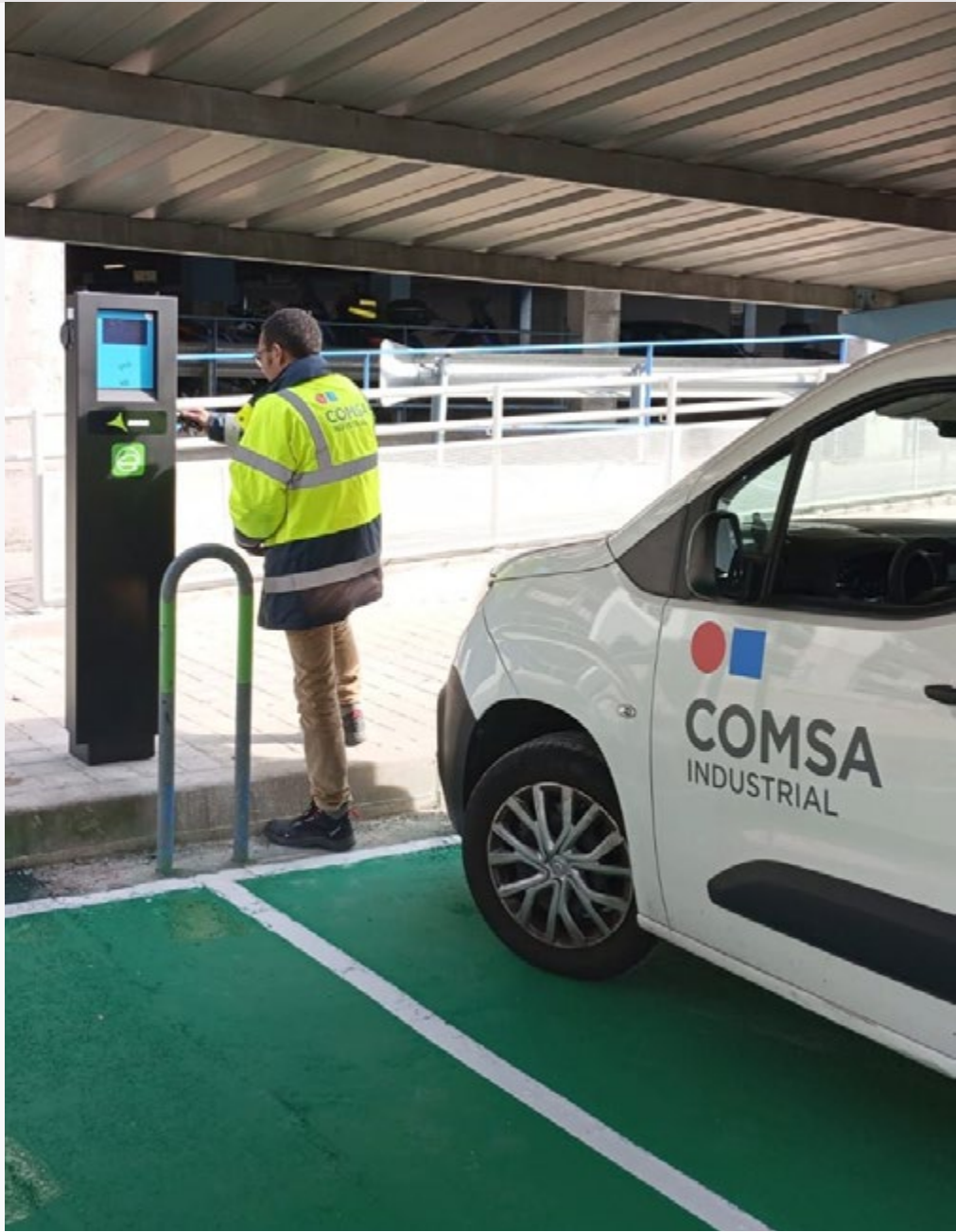
Charging points at Barcelona-El Prat and Madrid-Barajas airports (Spain). ▶
