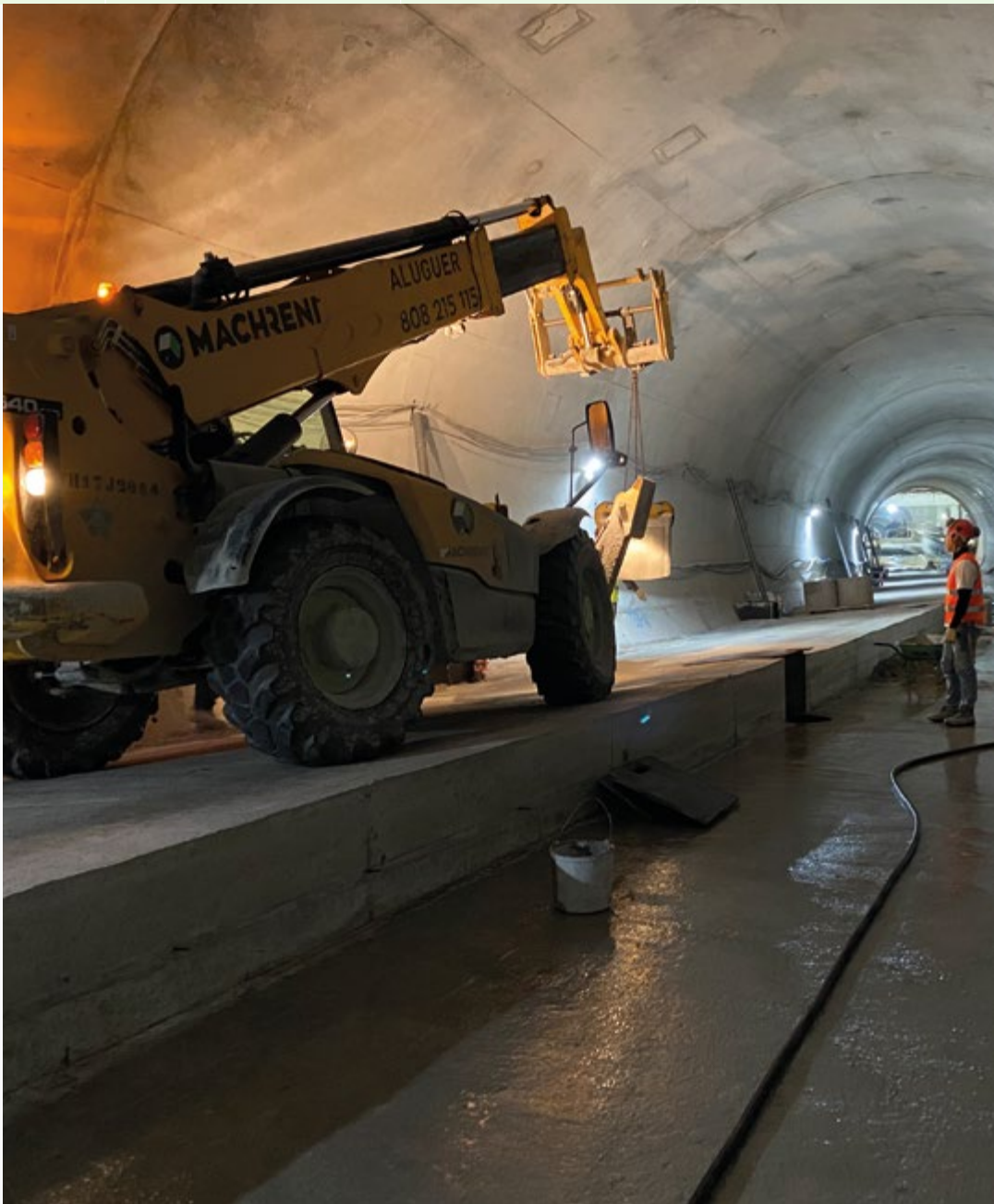
Expansion of the Amarilla and Verde lines of the Lisbon Metro (Portugal). ▶
