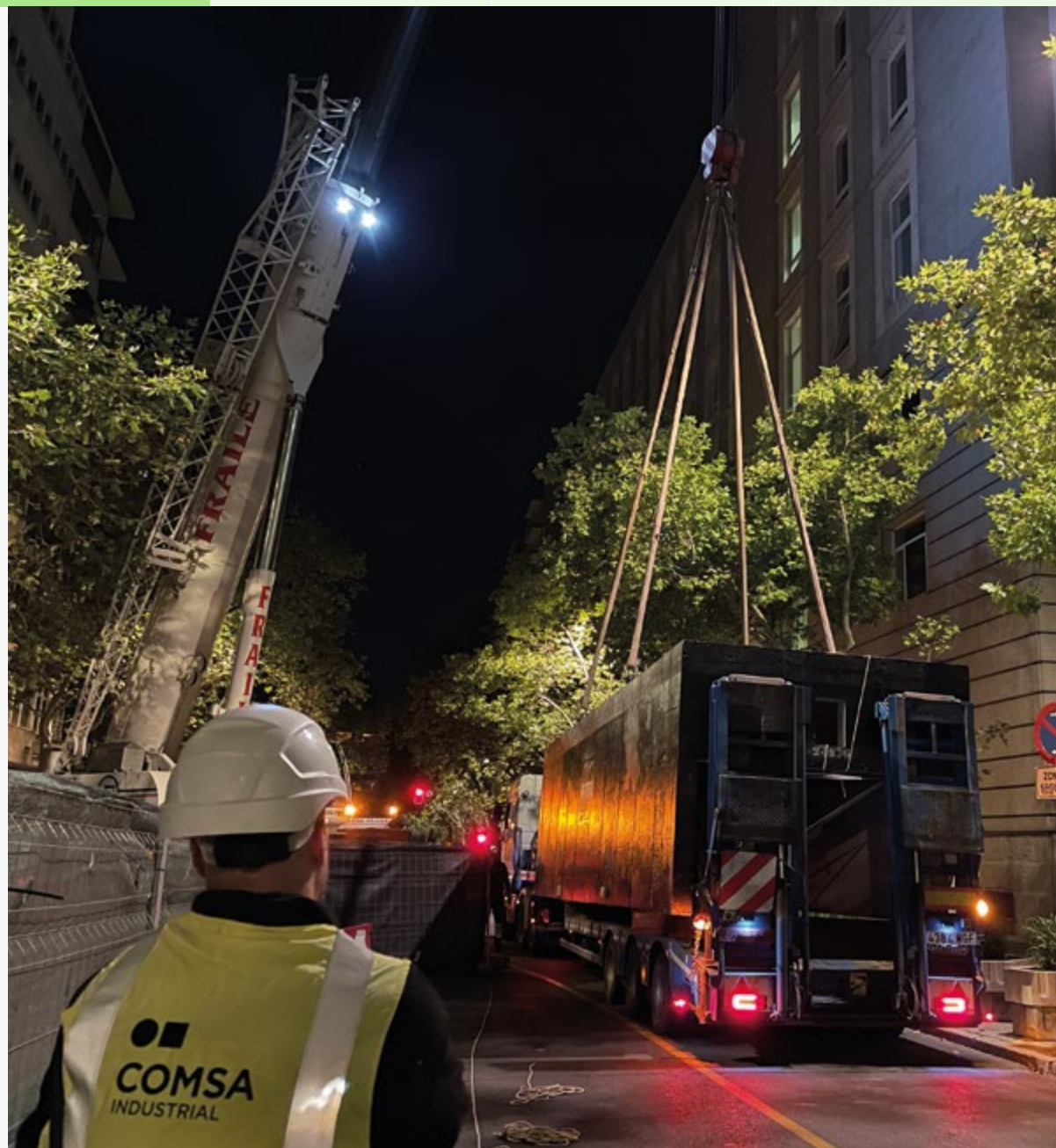
Relocation of the high-voltage line circuit Hortaleza - Azca in Madrid within the Unión Fenosa Distribución - UFD framework contract (Spain).
