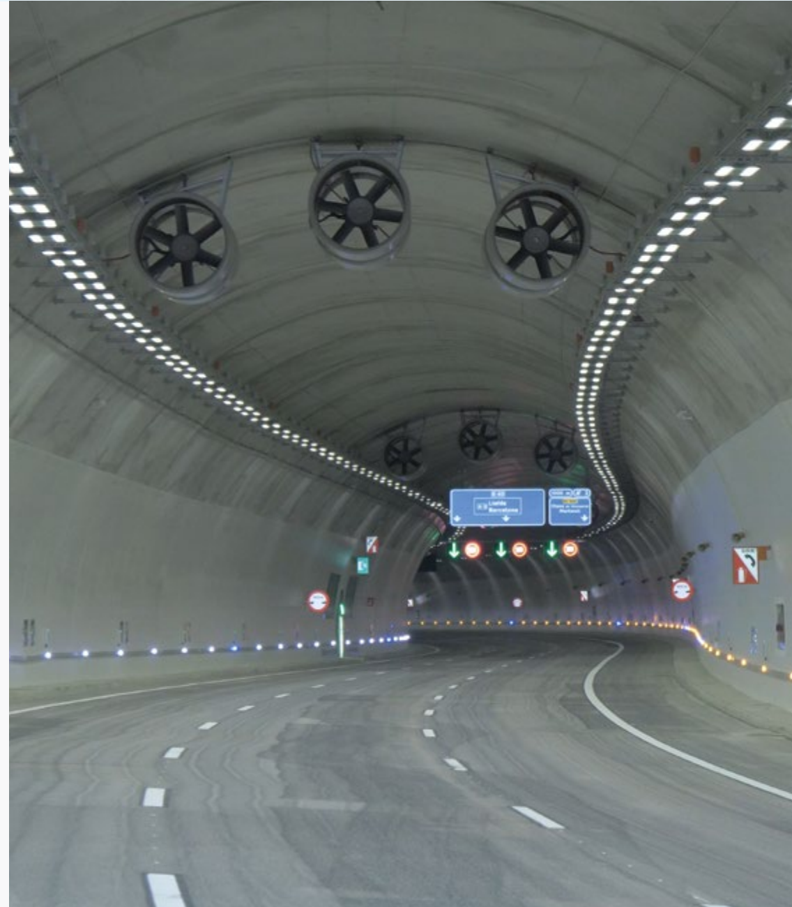
Facilities for the B-40 tunnel in Barcelona (Spain). ▶
