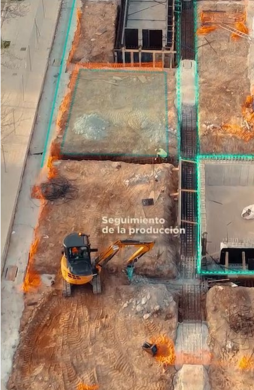
Real-time project tracking through the use of BIM methodology, which utilizes 3D digital models.
