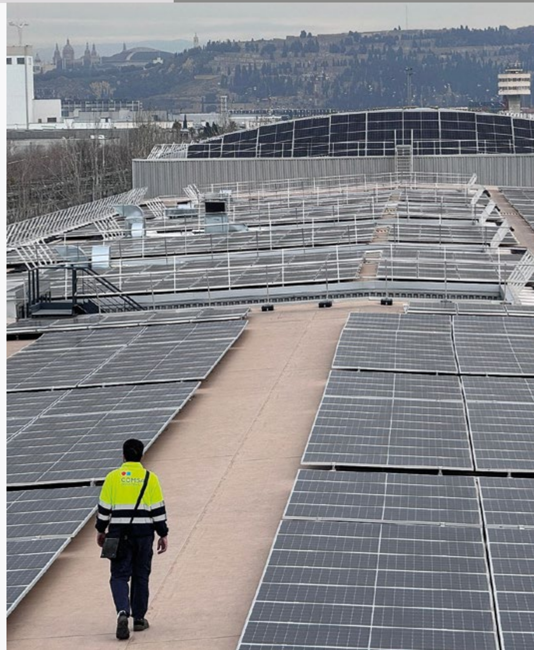
Photovoltaic plant on the roof of the L9/10 workshops of the Metro In Barcelona (Spain).
