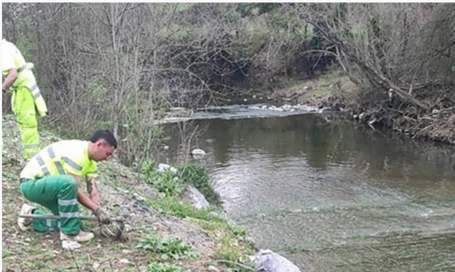
Planting of 3,102 trees, 2,243 shrubs, and the sowing of 46,635 m2 in the sanitation collectors project of the Alto Nervión basin in Araba and Bizkaia, Basque Country (Spain).
