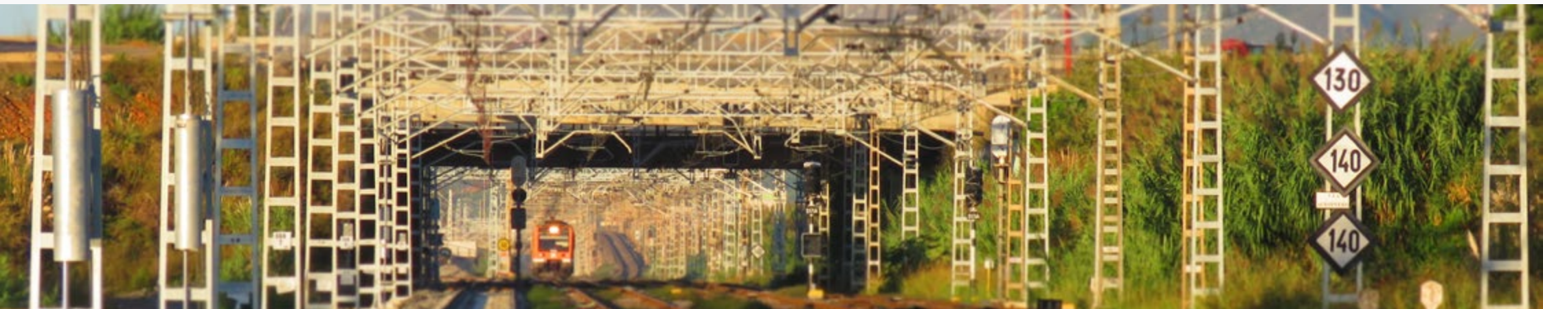
Renewal of the overhead line in the railway access to Terminal 1 of the Barcelona - El Prat airport (Spain). ▼
