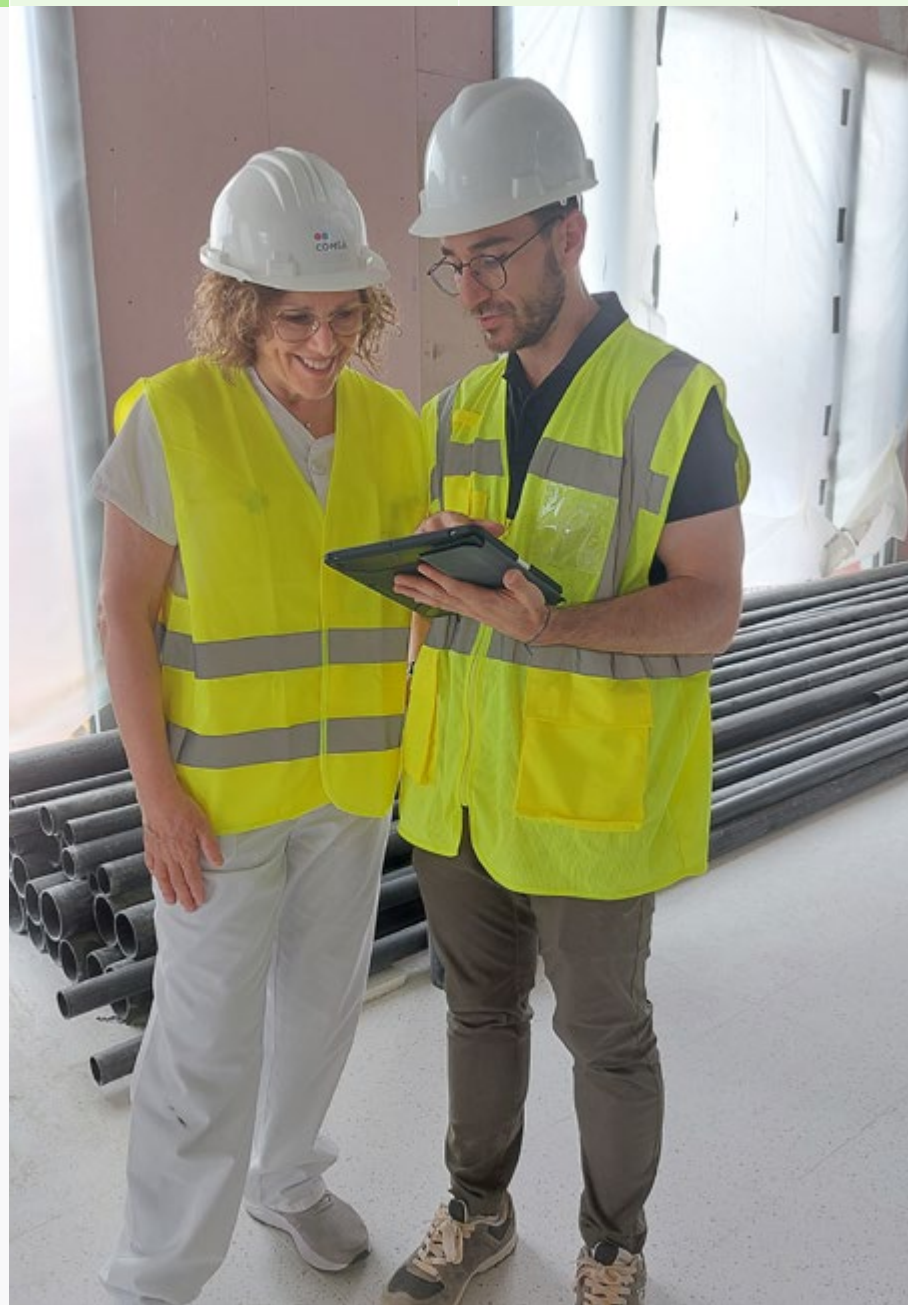
Digitalization in the building works of the Hospital Universitari Arnau de Vilanova in Lleida (Spain). ▶
