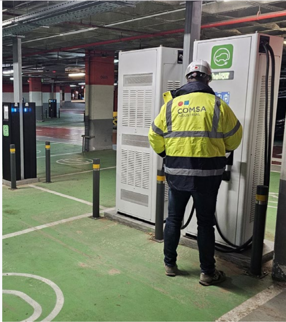
Installation of additional charging points for electric vehicles at the Barcelona and Madrid airports, using BIM methodology to optimize management throughout the entire life cycle of the installation (Spain).
