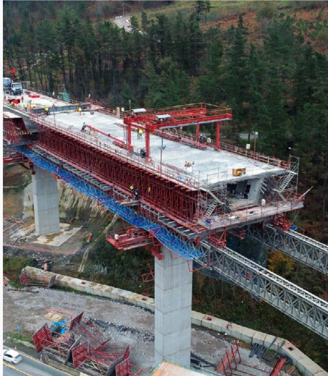
Construction of sector 3 of the Mondragón, Elorrio, and Bergara branch ▶ corresponding to the Basque high-speed 'Y Vasca' line (Spain).
