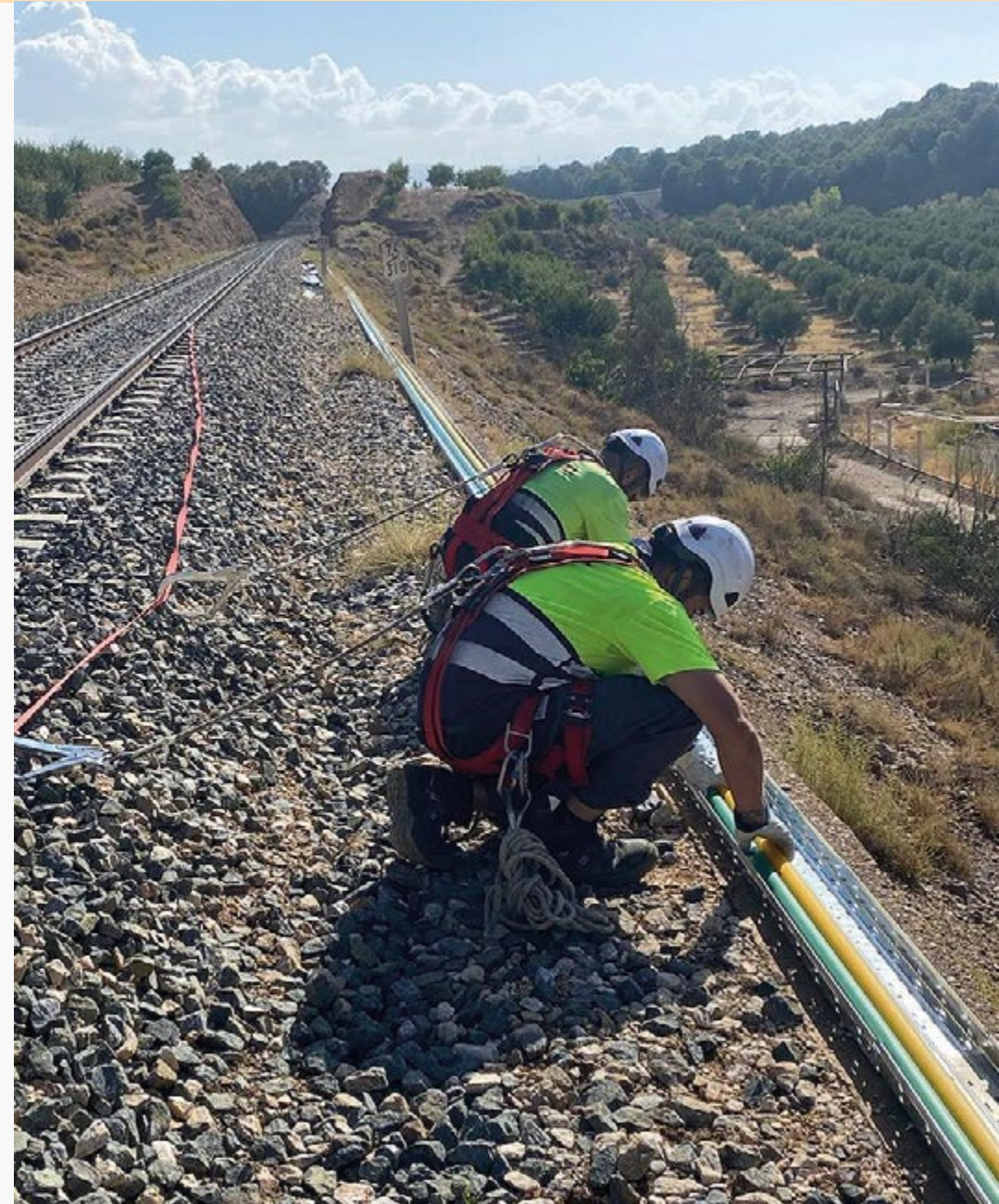
Renewal of communications infrastructure in the southern and central areas for ADIF (Spain).
