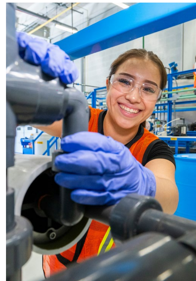
Water Treatment Equipment Installation at a Customer's Facility in Mexico
