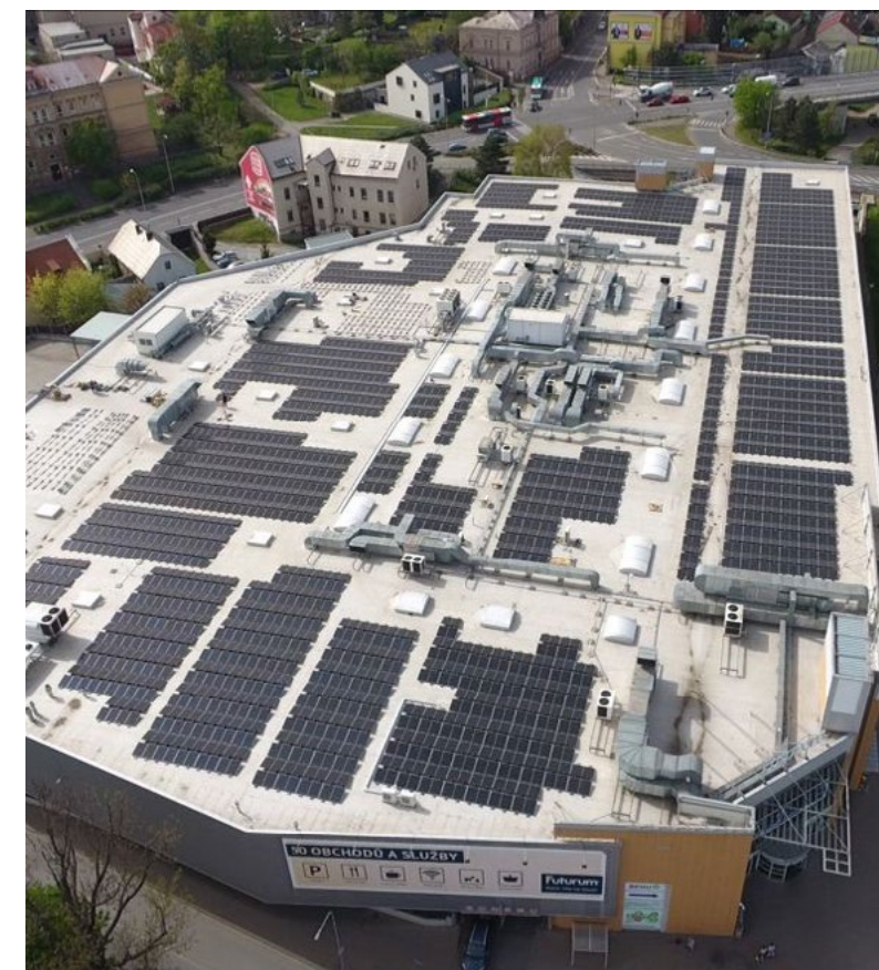
Rooftop solar panels, Futurum Kolín Shopping Centre, Czech Republic
