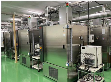
Equipment for conducting charge and discharge tests on batteries
