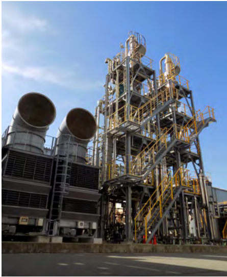
Ammonia stripping device at the Fukui Site
