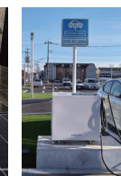
EV charging station installed on a parking lot
