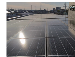
Rooftop solar panels (31.2 kW)
