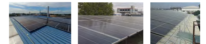
Newly installed solar power generating facilities From left: DIC Compounds (Malaysia), DIC Synthetic Resins (Zhongshan) and DIC Siam Chemical Industry
