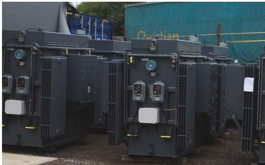
DORE's five new transformers
