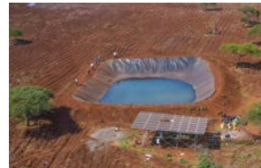
Solar irrigation system
