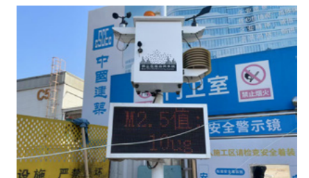
● Dust Monitoring Equipment
