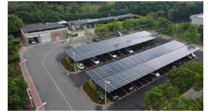
● Photovoltaic Power Station and Charging Pile Project at Xiamen National Accounting Institute
