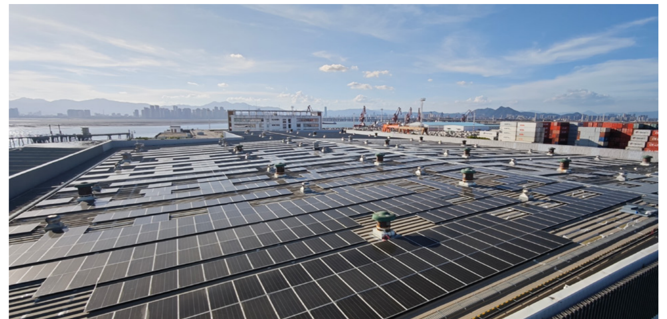
● Solar Power Station in Xiamen C&D Logistics Center
