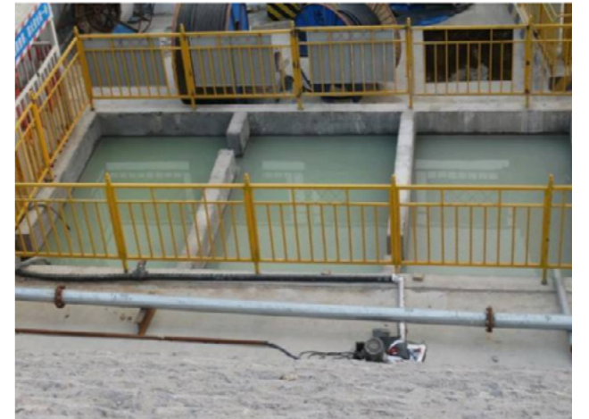
Sedimentation Tanks for Three Stages of Wastewater Treatment
