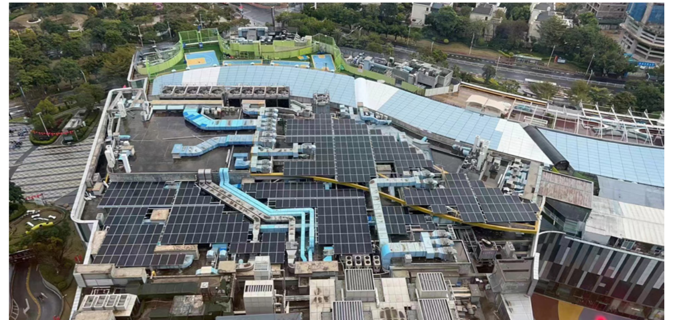
● Solar Power Station in Xiamen C&D OnePark
