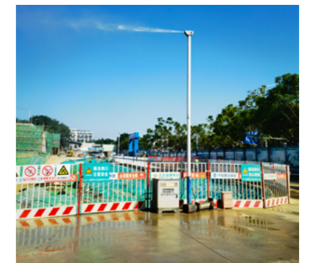
● High-Rise Sprinkler System
