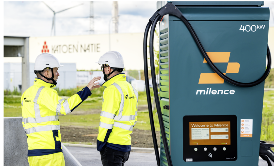
Near the port of Antwerp (Belgium), we have equipped an electric charging station capable of powering 20 lorries simultaneously.
