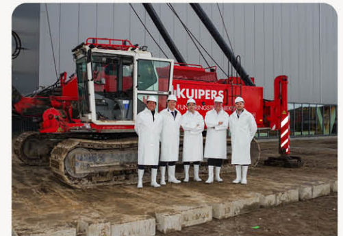
The new Crew Training Centre 'the Link' is taking shape to boost training capacity for future growth
