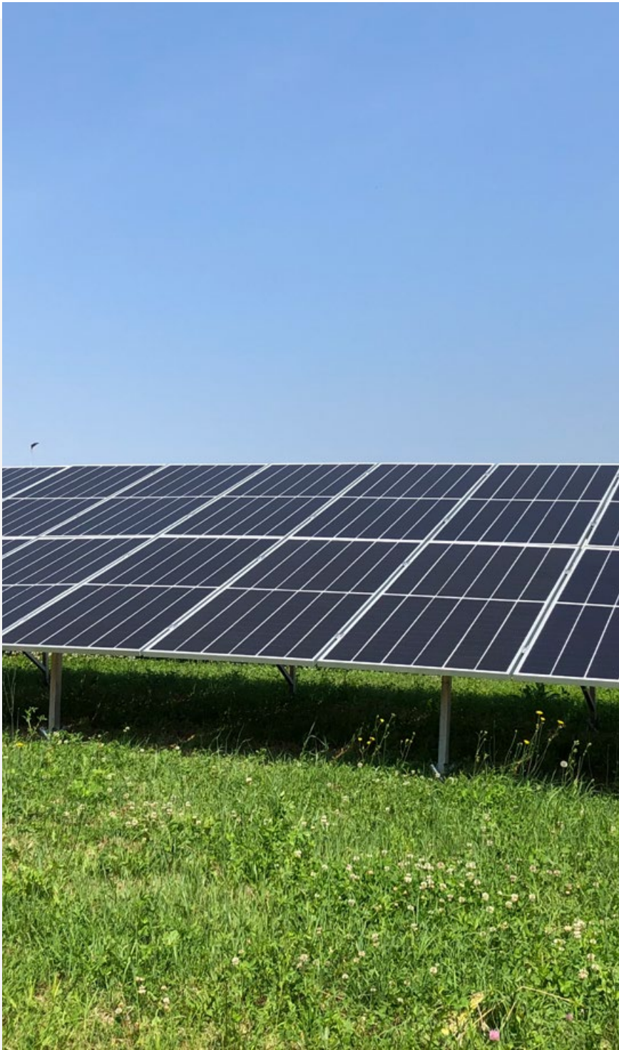
Solar park at Origgio site
