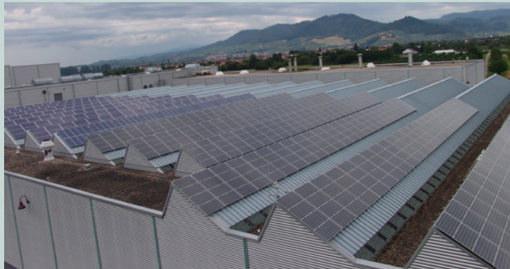
Further photovoltaic systems are gradually being installed on all available and suitable (roof) surfaces at Hansgrohe sites, such as here on a roof at the Offenburg facility.
