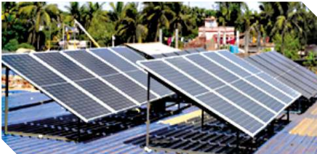
Total 3 MWp of solar installed at dealership facilities
