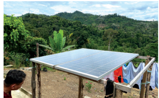
A solar panel installed at one of the houses in Kampung Paus.
