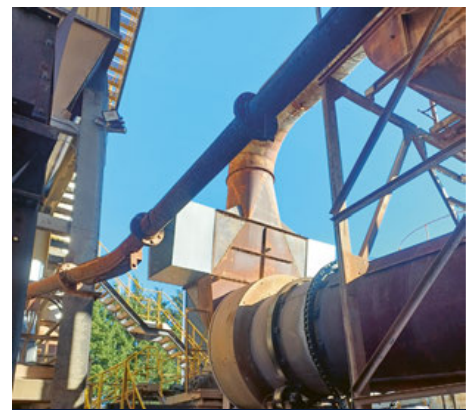
WASTE HEAT RECOVERY
