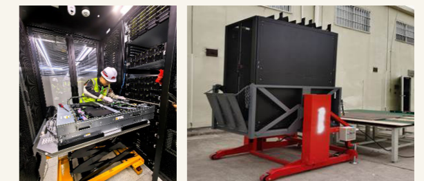
Delivery: A lifting platform assists with server installation and disassembly.
