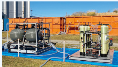
*2 PFAS water treatment system installed
