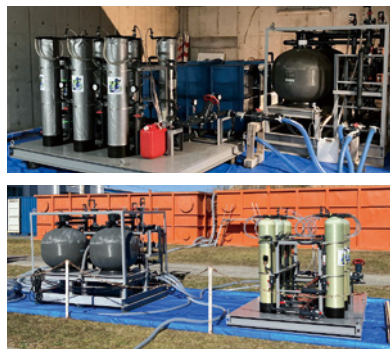
Water treatment system installed
