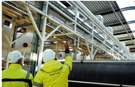
Inside the plant
