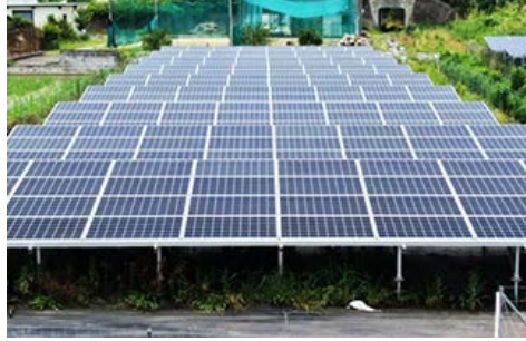
Off-site distributed power supply operated by Clean Energy Connect
