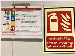
All Signs in Cambodian on Fire Prevention Facilities
