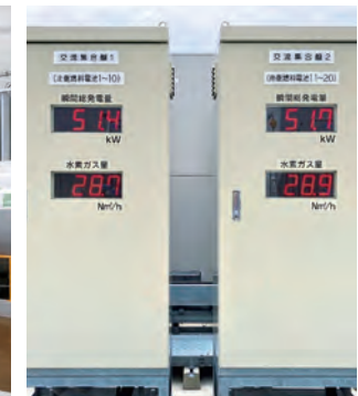
Pure hydrogen fuel-cell power generation equipment
