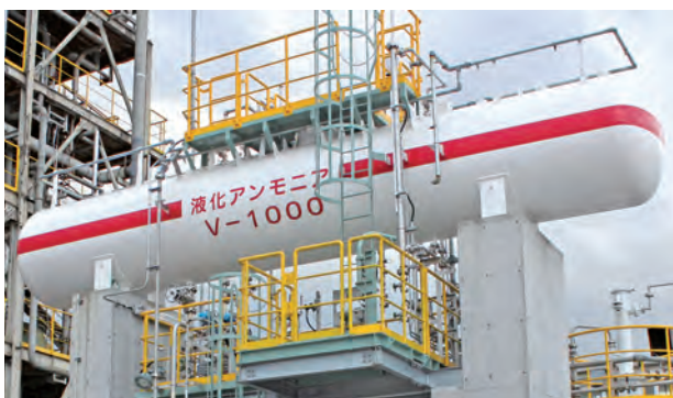
Ammonia supply facility
