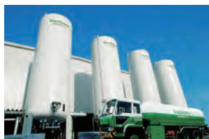
High-pressure gas supply facilities
