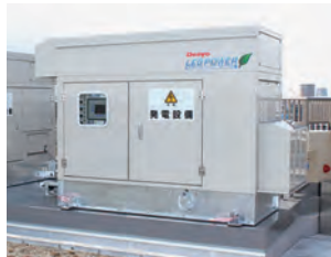
LPG emergency generator
