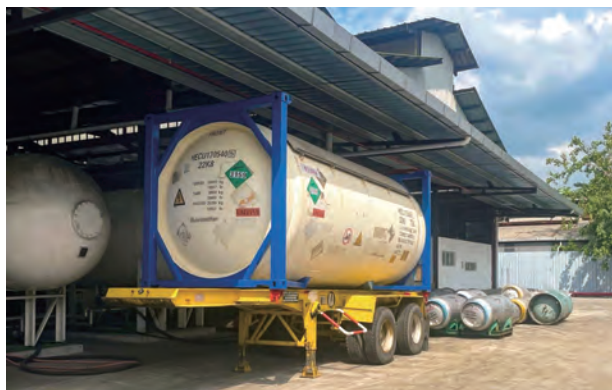
Refrigerant plant in Malaysia
