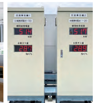
Pure hydrogen fuel-cell power generation equipment
