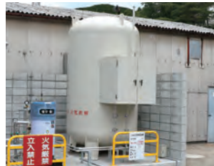
LPG supply equipment
