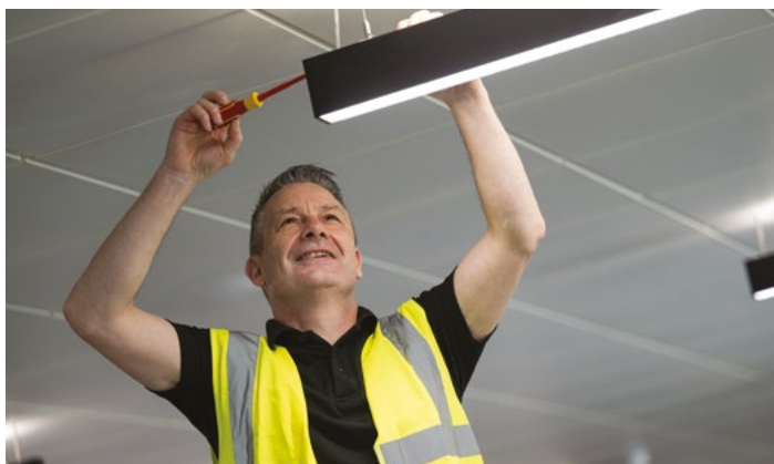
Enhancing energy efficiency: A team member installs new LED lighting as part of our commitment to rolling out this technology across our entire property portfolio.
