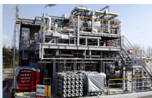
Ammonia synthesis pilot project facility (Fukushima)
