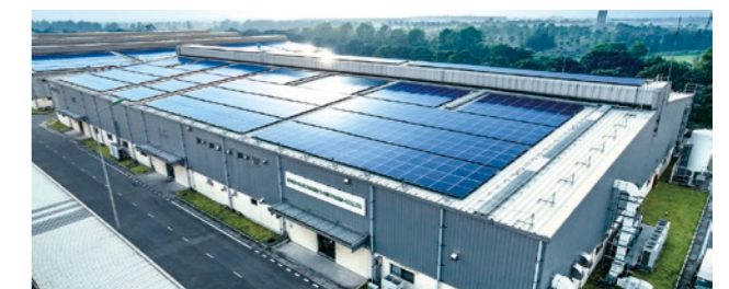
Solar panels installed at a facility in Vietnam
