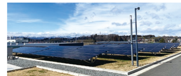
Solar panels installed at Fukushima Site
