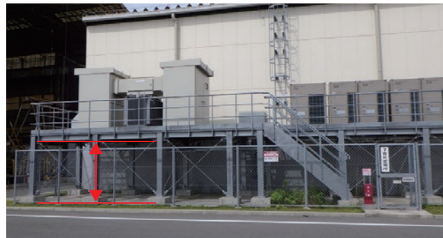
A substation at the Kobe Works
