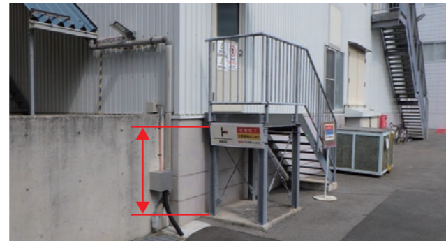
A power receiving station at the Kobe Works
