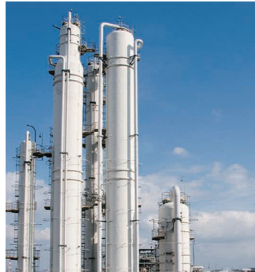
Distillation columns at the chemical plant (Credit: ENEOS Materials Corporation)
