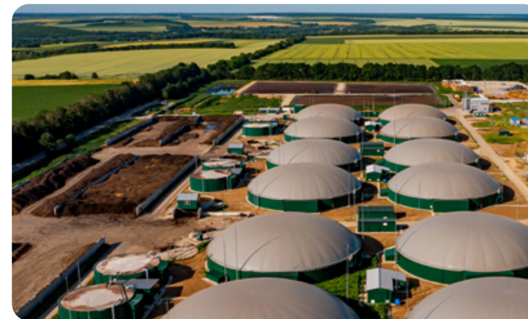
Renewable natural gas plant
