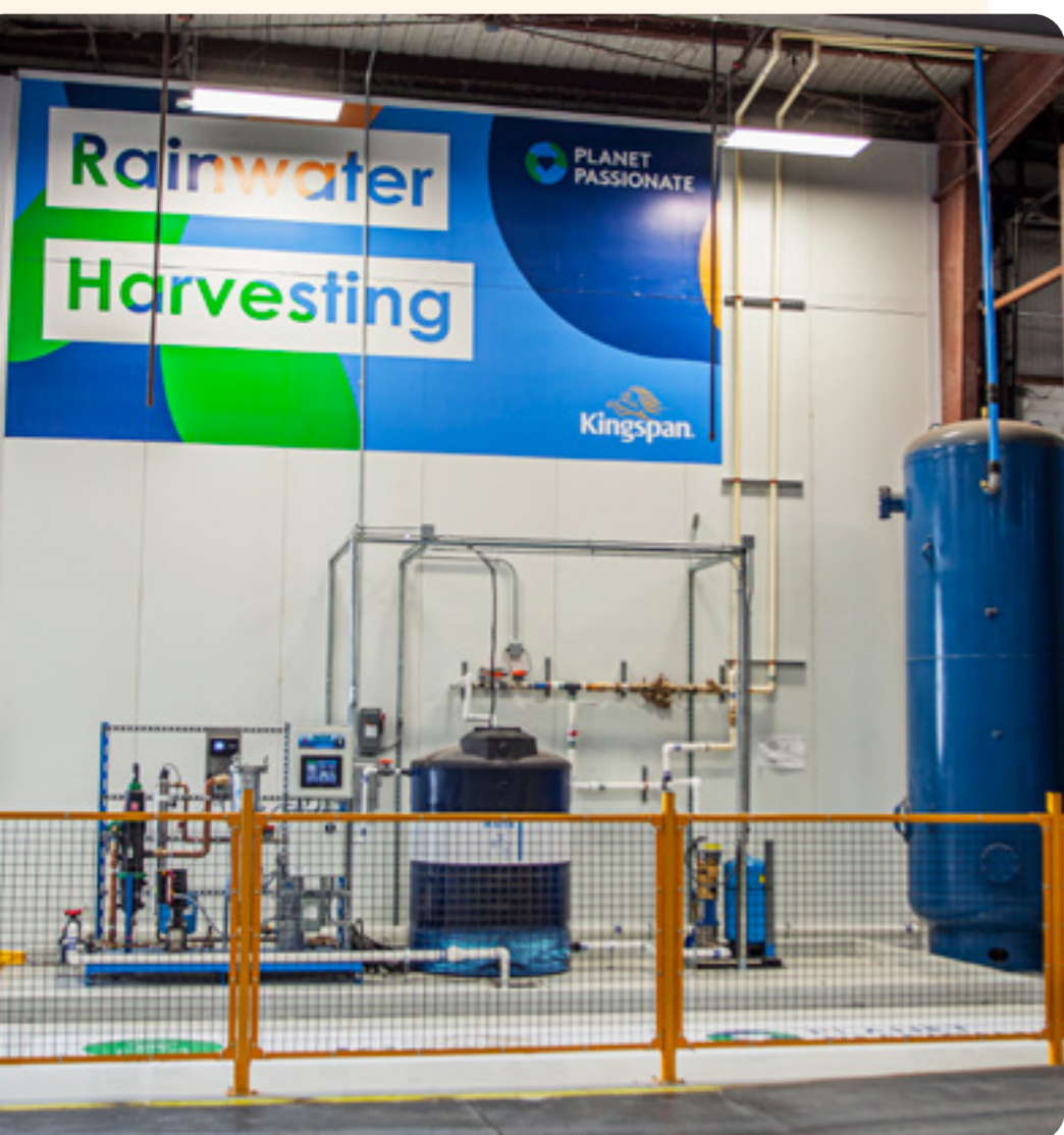
Rainwater harvesting in DeLand, FL
