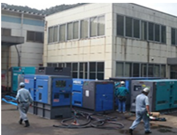
Disaster recovery support (lending electric generators)
