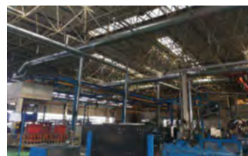
An example of measures to meet regulations in China (Daikyo Machinery Shandong Co., Ltd.: Installation of a welding fume dust collector and exhaust air ducts)
