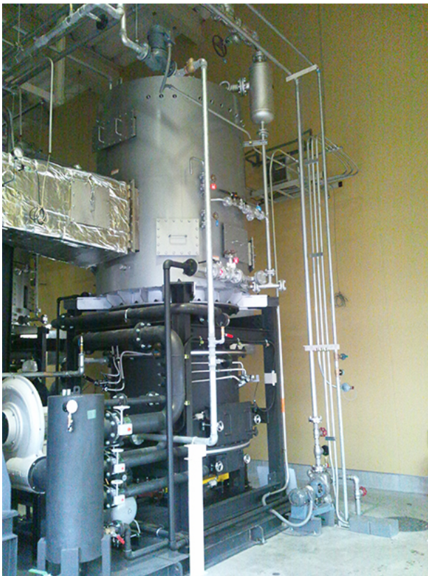
Wood biomass boiler
