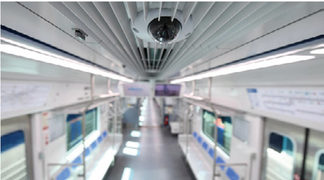
CCTV Installed in Metropolitan Subway
