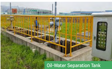
Oil-Water Separation Tank
