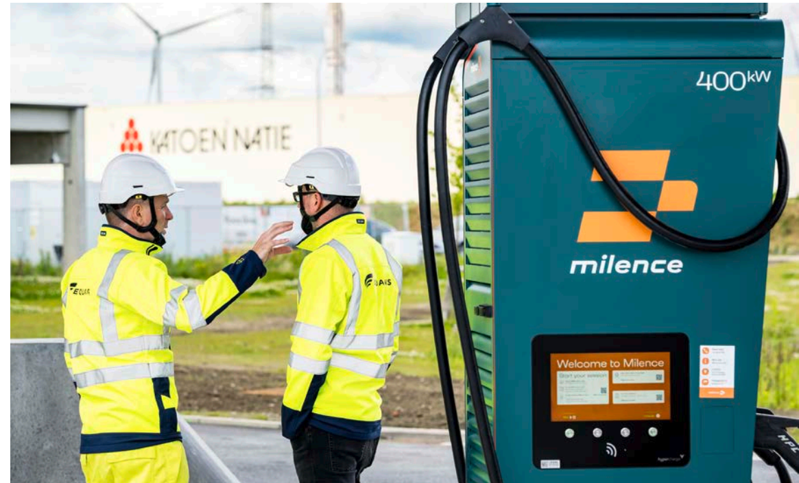
Near the port of Antwerp (Belgium), we have equipped an electric charging station capable of powering 20 lorries simultaneously.
