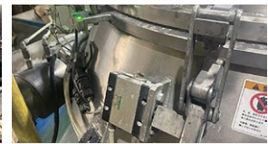
The opening of the mixer is equipped with a limiter switch, which prevents people from approaching while the mixer is in operation.
