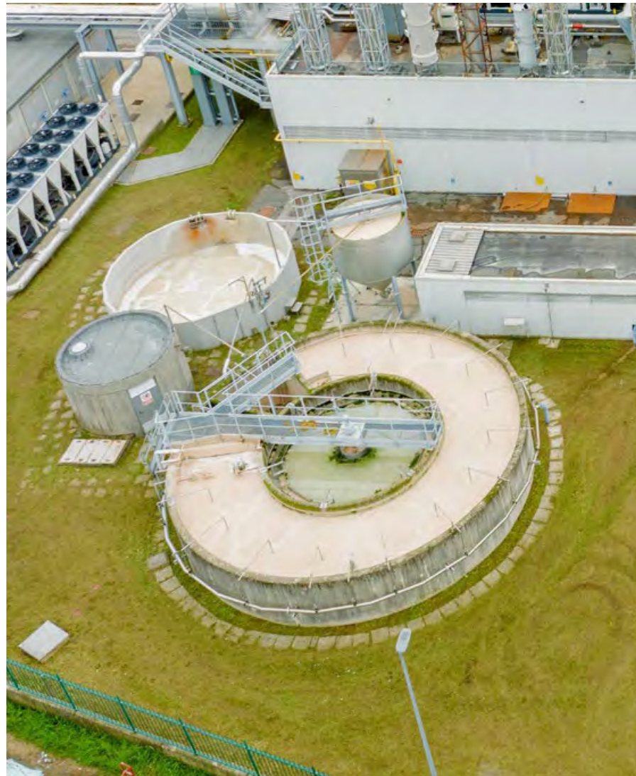
Waste water treatment Origgio site
