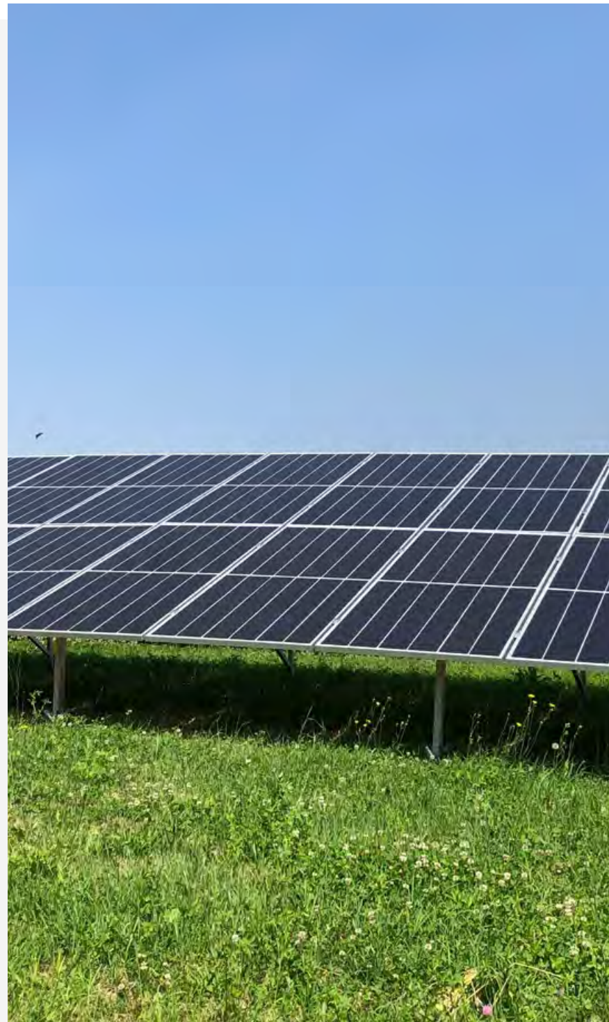
Solar park at Origgio site
