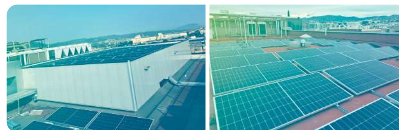
Photovoltaic panels on the facade and rooftop in Sant Joan Despí
